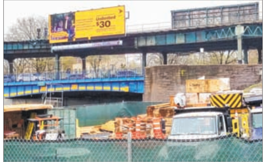
Work has begun on the Westchester Avenue Bridge over the Hutchinson River Parkway to make the bridge higher and roadway safer to prevent accidents. Arthur Cusano
