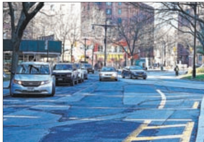
The streets of Parkchester are the worst in the Bronx, according to a report put together by the Independent Budget Office using NYC DOT data
