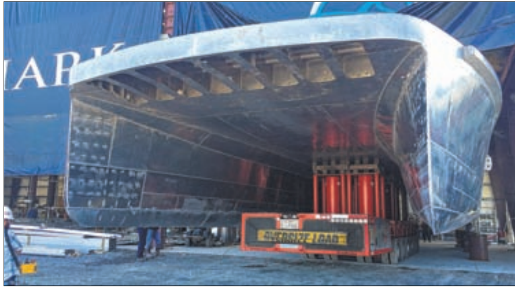
One of the ferries under construction that is part of the planned citywide expansion that includes the Soundview stop. Photo courtesy of NYCEDC
