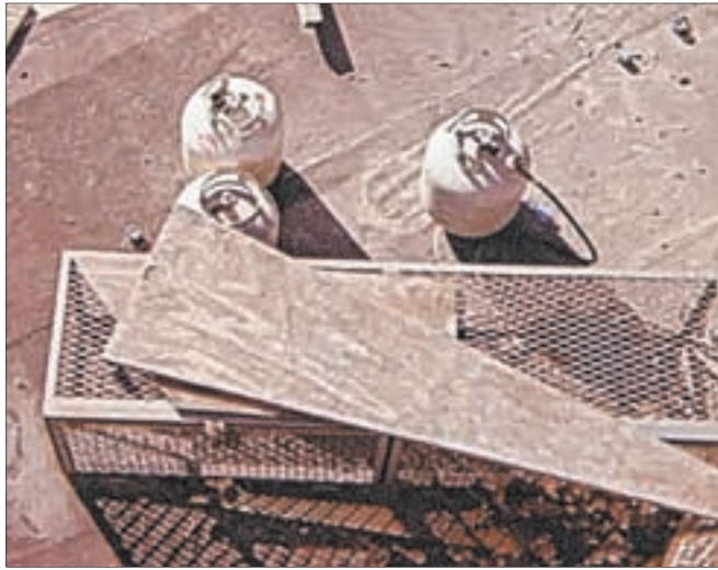
Propane tanks were seen sitting on top of Vivero Macca Live Poultry's roof. Photo courtesy of Robert Gerola
