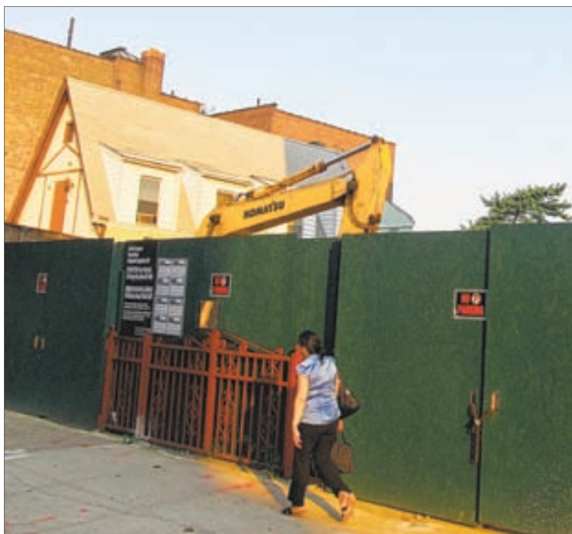
Work fences on apartment building projects, like this one in Pelham Bay on Buhre Avenue, dot the landscape in some communities, raising overdevelopment concerns once again.
