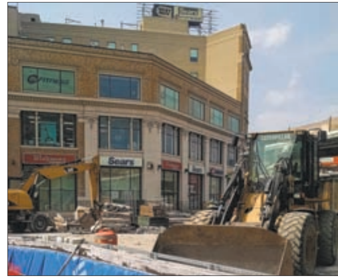
Fordham Place, formerly known as 404 E. Fordham Road, will be the new home of a Macy's Backstage after Sears occupied the building for nearly eight decades. Surrounding construction is part of the Fordham Plaza Reconstruction Project. Community News Group / Steven Goodstein
