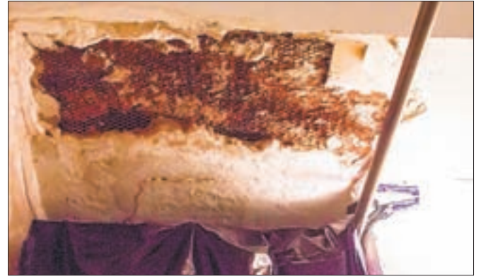
The ceiling collapsed in Melody Ruiz's bathroom after years of leaks and patch jobs. Photo by Silvio Pacifico
