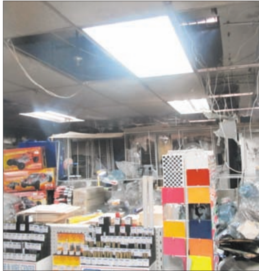
A view of the damage inside Bruckner Hobbies.
