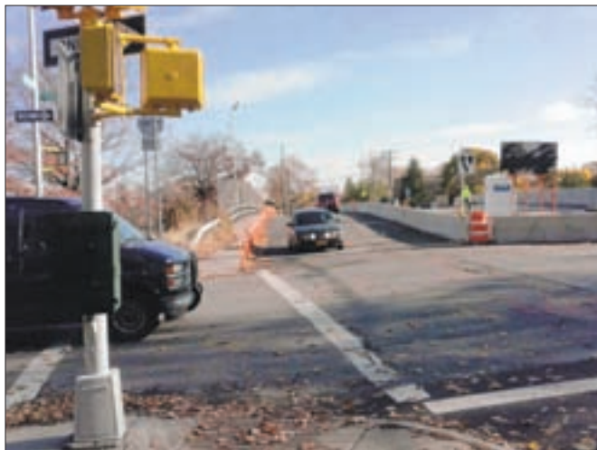
Lafayette Avenue Bridge is one of three local area overpasses undergoing renovations. Community News Group / Robert Wirsing
