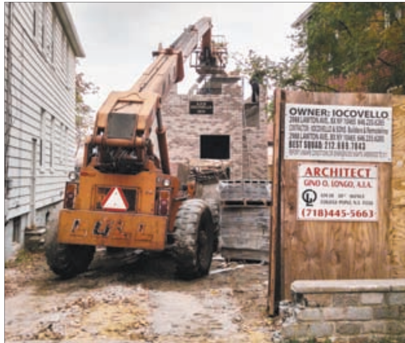
The thin house on 848 Revere Avenue, resumed construction on Monday, November 3, after it was halted for over three months by the NYC Buildings Department.
