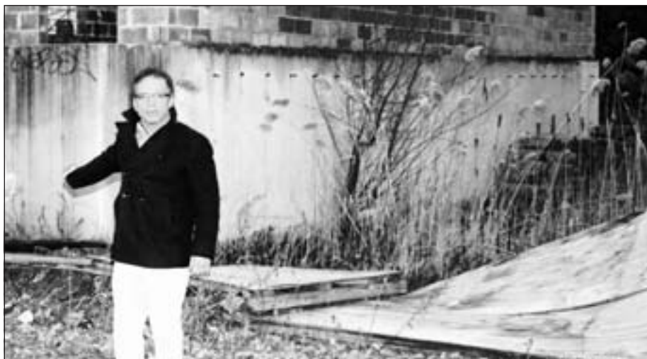
Councilman Jimmy Vacca points to the fallen fence at 817 Hollywood Avenue before repairs were made. Photo courtesy of Councilman Jimmy Vacca
