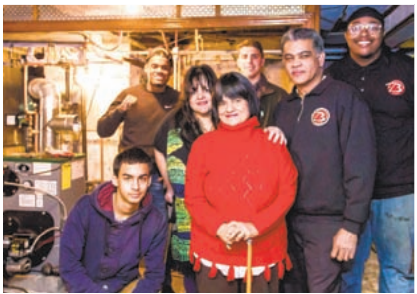
(l-r) Justin Gonzalez, Joshua Diaz, Milagros Orizal, her mother Gladis Medina, Eddie Puncar, Pete Gonzalez and Tyree Jordan stood near the newly installed boiler.
